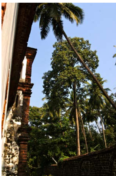
Figure 5: Palm Trees Growing and Pushing Church in Decay (Goa, India)
